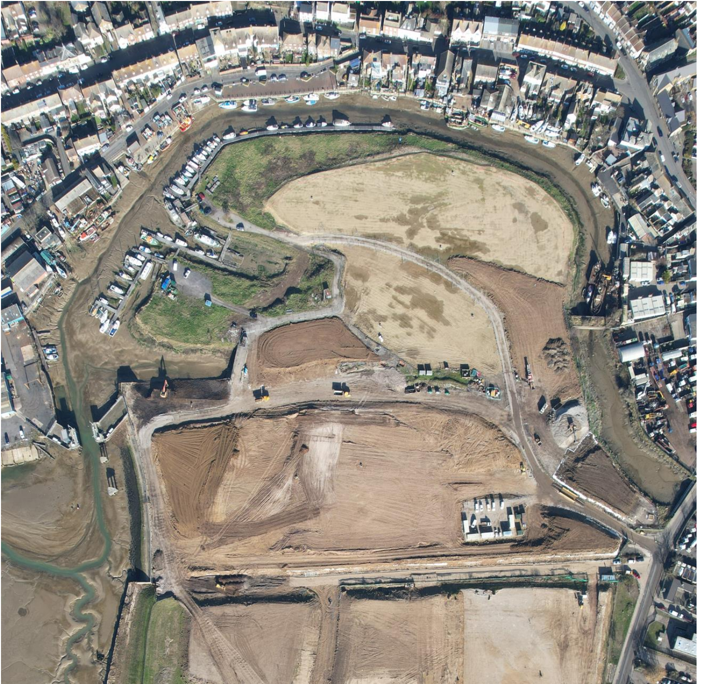
Klondyke site- works almost complete (Twyfords site to the south of the road)
